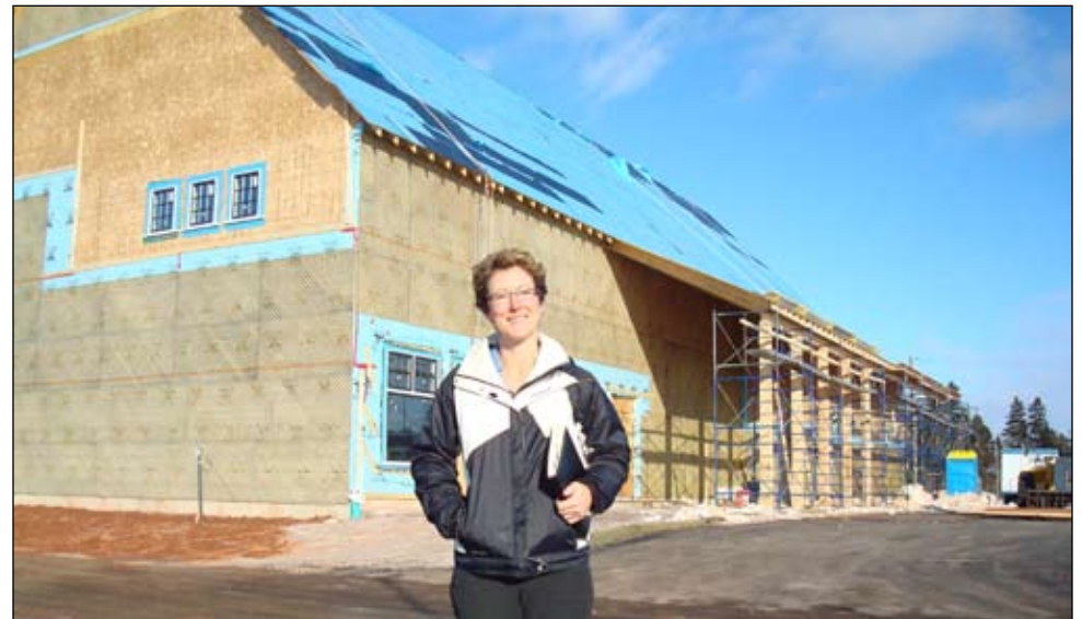
Ann Worth, Director of Operations for COWS, in front of the COWS CREAMERY under construction at the North River Causeway. The new building is scheduled to open in May.
